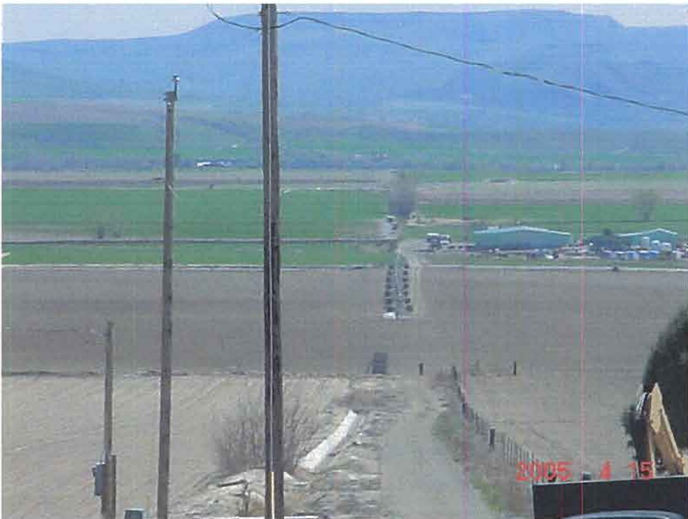
Sunset Valley Irrigation Enhancement Project Photopoint #2: Pipeline and Pivots 4/15/05 (monitoring)
